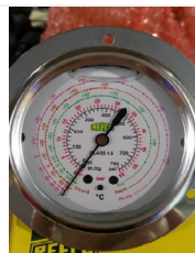
Example of empty (loss of refrigerant)
