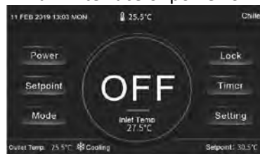
Main interface of power-off
